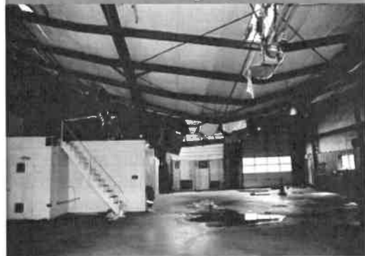
Figure 5.6 — As a result of a storm, this station roof buckled under the excessive water weight.
