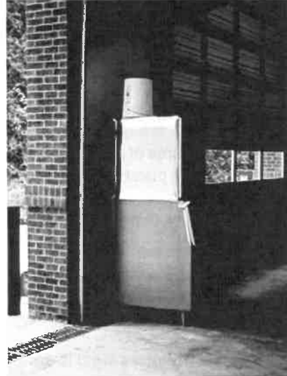
Figure 6.15 — Ice machines should not be placed in areas subject to exhaust or other contamination.
