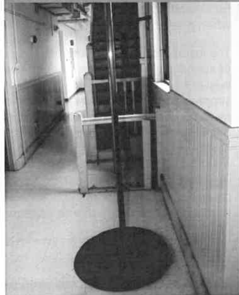
Figure 5.5 — There should be protective padding at the bottom of a slide pole.
