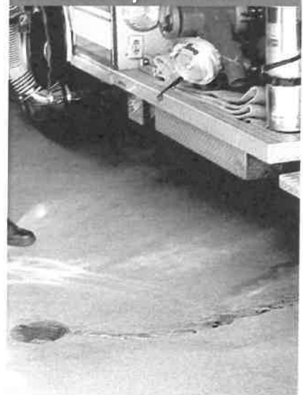
Figure 7.8 — Improper placement of apparatus floor drains create wet spots that will cause slips and falls.
