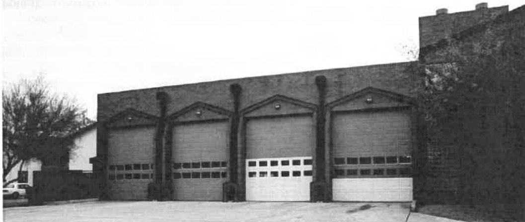
Figure 4.10 — The different colored panels on two of these roll-up doors indicate that they have been damaged in collisions.
