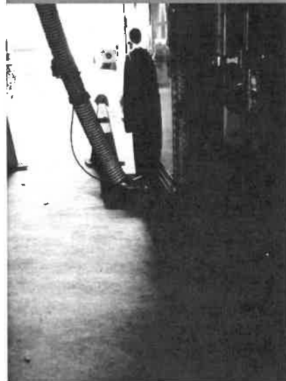
Figure 1.2 — A typical apparatus exhaust system connection.
