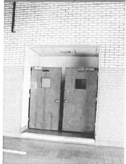
Figure 7.1 — One door leads from the kitchen and one from the dayroom; both are hinged on the wrong side. There is also a hazardous step-down to the apparatus bay.
