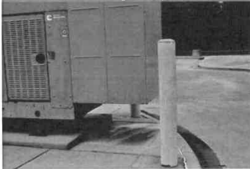
Figure 7.4a — These bollards protect the station's emergency generator.
